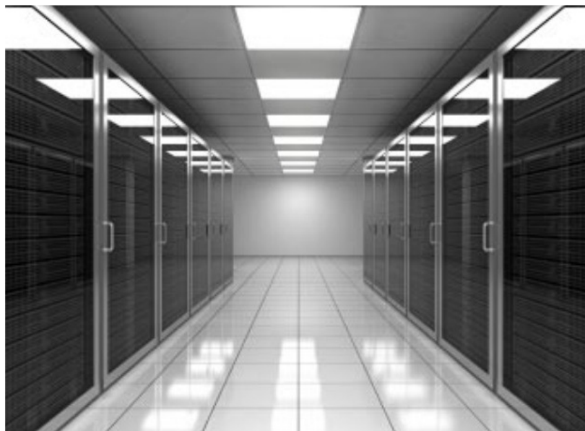
Inside Cloud9 Real Time's data center
